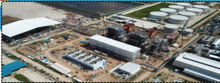
Biomass Power Plant
